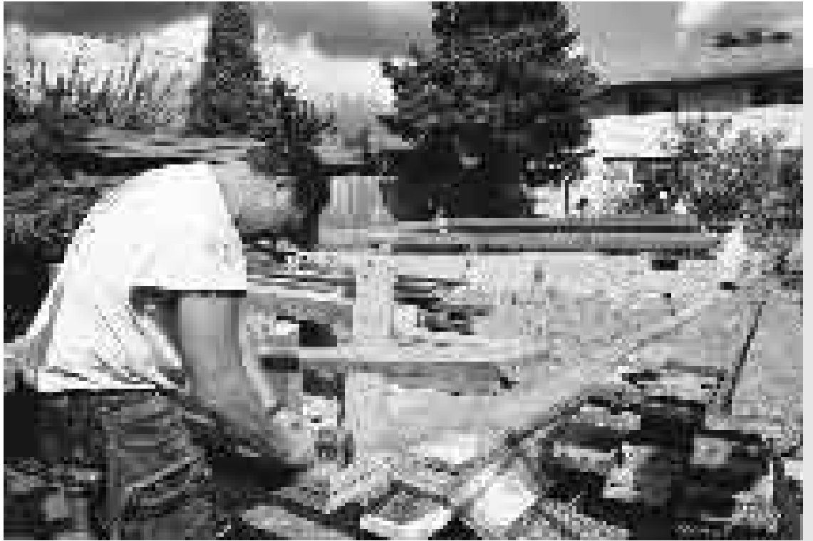
A framer cuts the first floor joists (made with reused lumber) for a Portland, Oregon duplex made almost entirely of reused wood. Much of the lumber for the 1,730-square-foot house came from an old grain mill. Photo courtesy SCNW.
